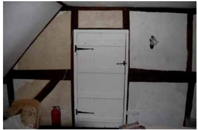
Figure 4. The doorway inserted into the upper part of the cross-frame between the hall and parlour bays, which avoided the need to 'duck' under the tie beam to move between the upper floor rooms.
