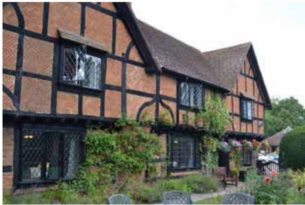
Fig.3. The south range showing the very uniform brickwork above the jetty. This is in contrast to the brickwork elsewhere which exhibits much more variation, and wider bricks, and probably indicates the major restoration work that was undertaken.
