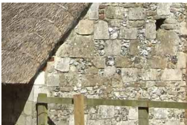
Fig. 2. The walls of the great barn at Hensting Farm are mainly composed of shaped stone blocks.
