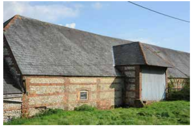
Fig. 25 building 8. The west-facing porch of the brick and flint barn, which was probably built at the end of the 1830s.
