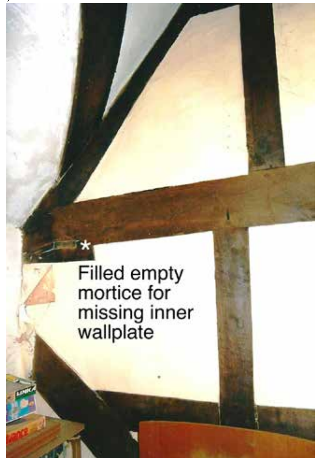
Fig. 2. The filled mortice for a missing inner wall plate in a tie beam at one end of the hall at Abbey Farm, Mottisfont.
