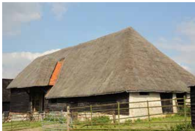
Fig. 3, building 4: A 5-bay thatched threshing barn built in the early 18th century.
