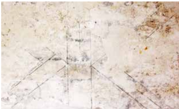
Fig. 2. Wall painting at Park Farmhouse.
