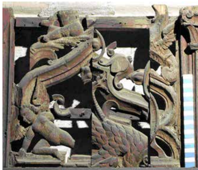
Fig. 3. Hospital of St Cross, Winchester. Bay 3 in the upper tier frieze as photographed in 2007 (scale 200mm). Photograph: Nicholas Riall.
