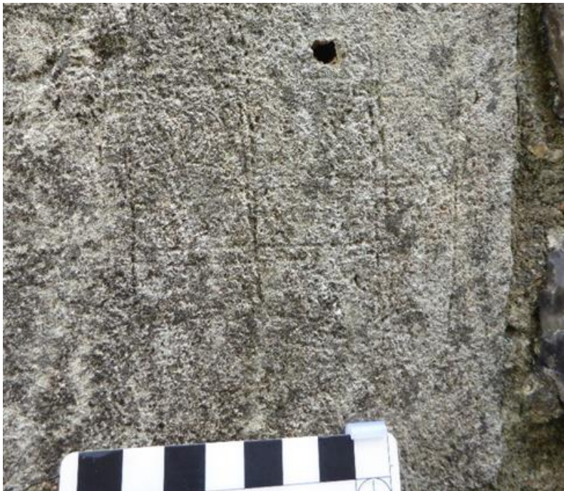
Fig 19. Tower. Northwest buttress. Grid pattern
