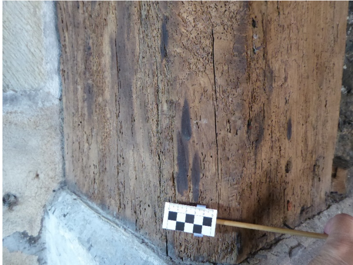
Figure 5 Taper burn marks in tower
