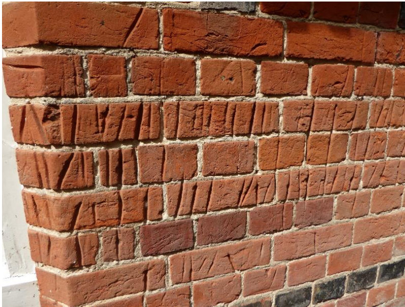
28 "Pencil" sharpening marks on brick wall of former village school adjacent to church
