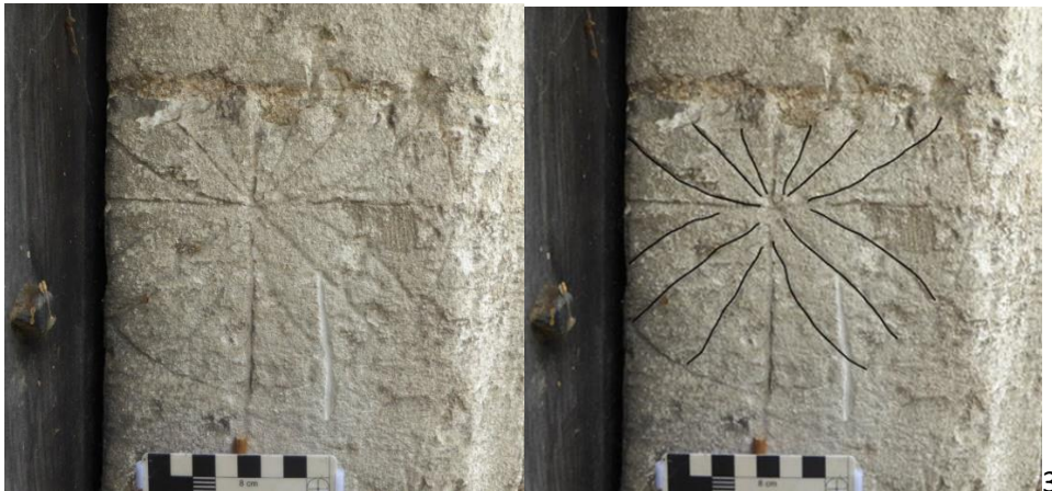
11 South side of west door. 2 views of circular device with quatrefoil, with annotated image on rhs. Possible consecration cross
